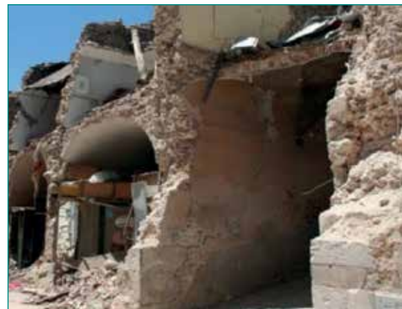
Fig. 6 – Example of overturning of perimeter wall.
